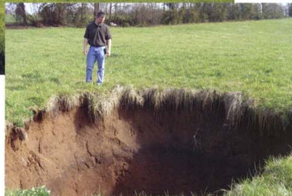
Collapse off Cemetery Road
